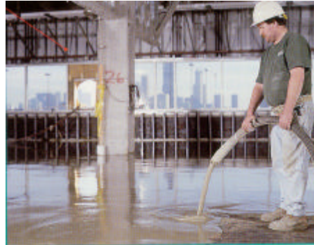
Rapid Floor Ultra saves time with high-volume application equipment capable of pumping 1,000 to 30,000 square feet (93 m 2 – 2787 m 2 ) in one workday.
